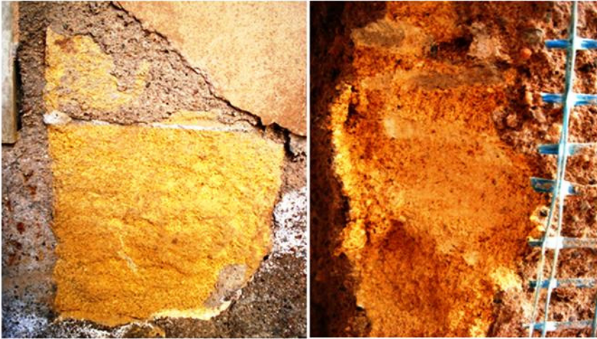
Figure 5: Mortar coating (left). View of the support (tabaire stone) and presence of salts on the surface of the cement mortar (right) (Lasheras and Lanzón [17]).
